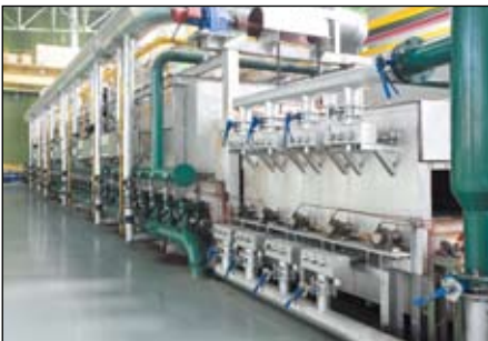
固溶炉 Solution Heat Treatment
