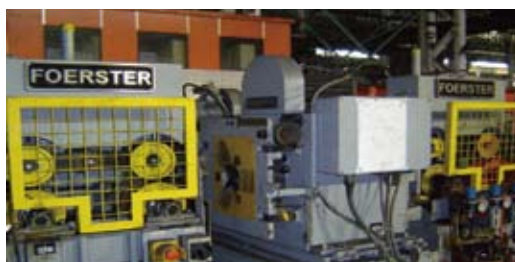
A、B、C、D线棒材漏磁探伤设备 magnetic flux leakage testing equipment for wire and bar installed in Line A, Line B, Line C and Line D
