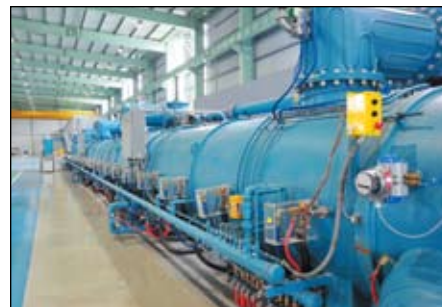
真空炉 Vacuum Furnace
